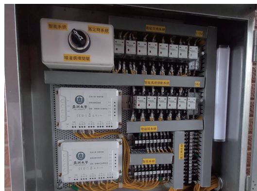
Fig. 10. (Color online) Smart switch panel to operate actuator of water valve controller.
