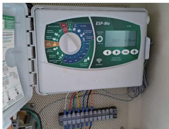
Fig. 13. (Color online) Previous sprinkler control system.
